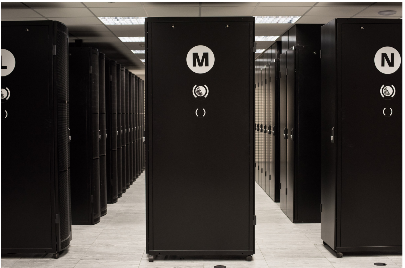
Photo: Installation of racks in our Namesco Data Centre
