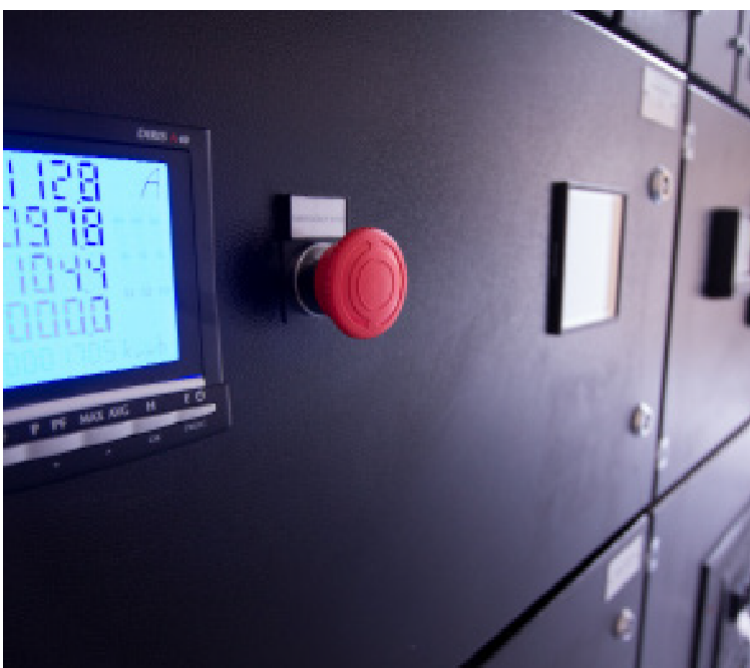
Photo: Switchgear on the "A" side compartment at our Namesco Data Centre
